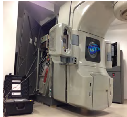
The B160R11 service unit is adapted to the requirements of small gas compartments. The photo shows the device during service works on an irradiation unit.
